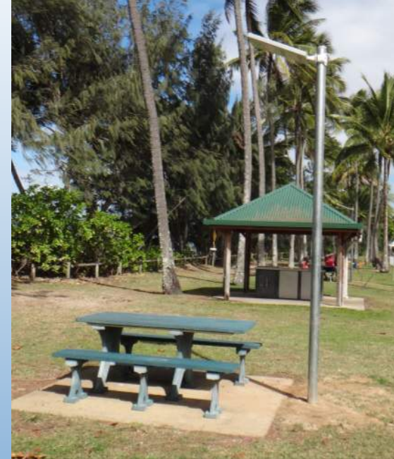
Solar light panel
