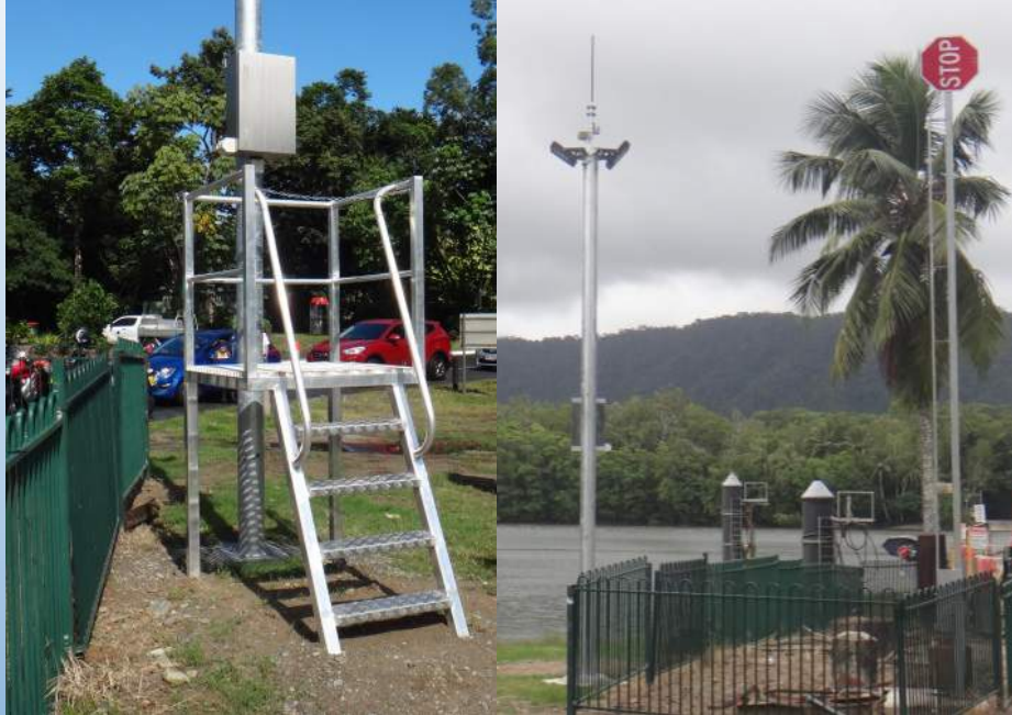
Ladder & light pole
