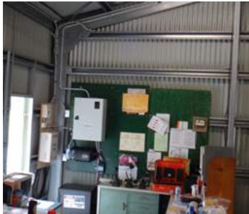
(Above) Diwan SES New Solar inverter
