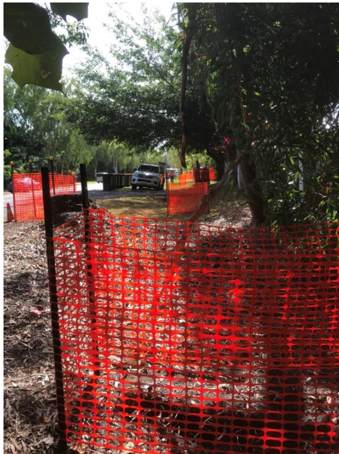
Image: Preparation to under bore for lighting power lines on Barrier Street Ordinary Council Meeting - 30 April 2024
