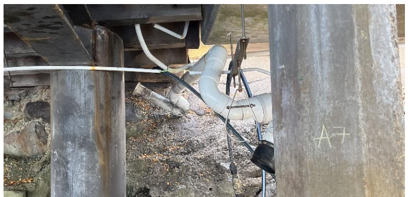
Images: Damaged pipes beneath the Sugar Wharf
