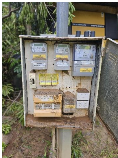
Images: Daintree Ferry Ticket Office and power supply after flood Ordinary Council Meeting - 30 April 2024
