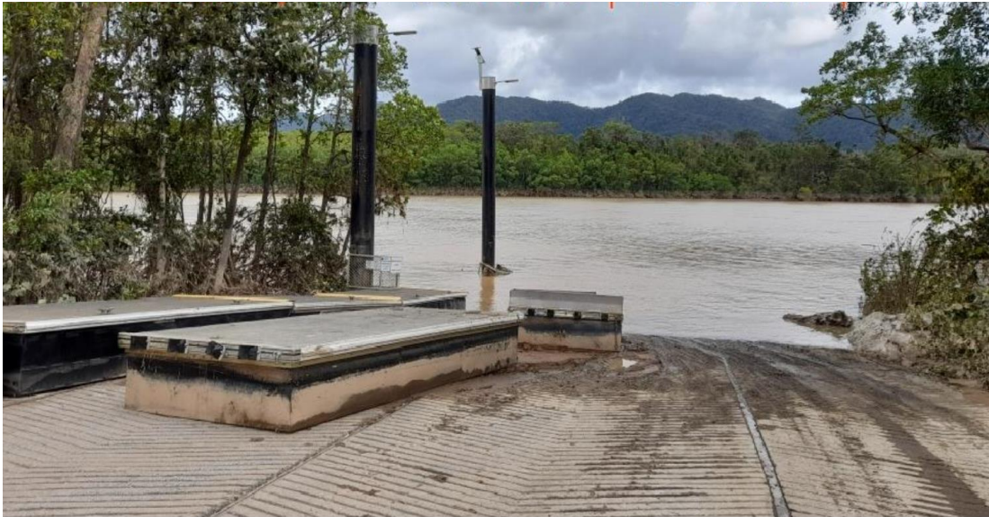
Image: Post TC Jasper damage to the floating walkway – Lower Daintree boat ramp
