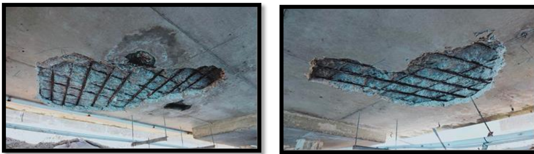
Pic 001 & 002 [ concrete areas that let go during repair work]
