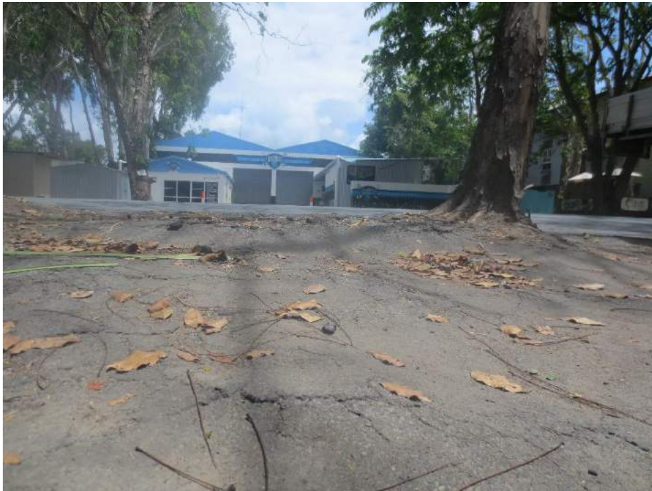
Image 2 – Impact of surface roots on parking and roadway
