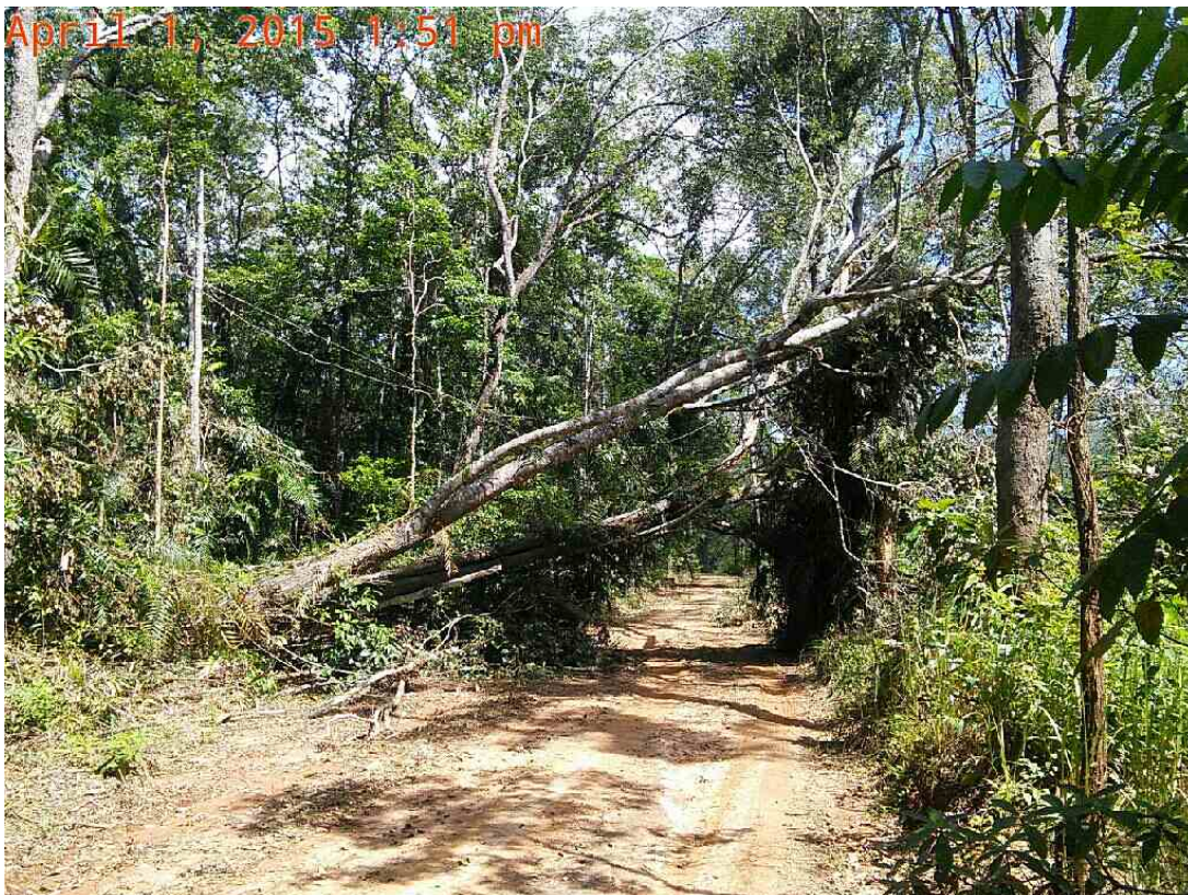
Typical damage due to Cyclone Nathan – China Camp Road
