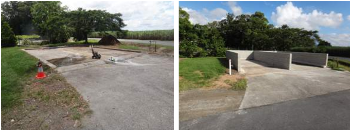
(Above) Two Views of the mulch bay (before and after the project was completed)
