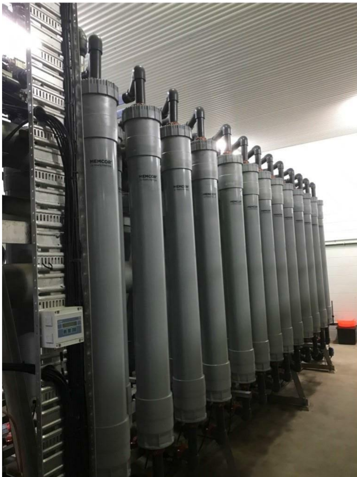
Figure 7. Memcor membranes at Mossman/Port Douglas WTP
