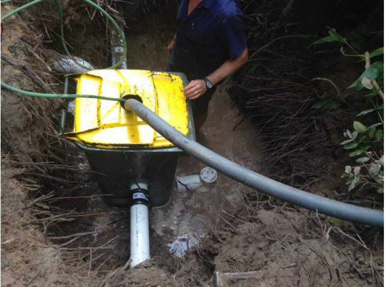
Innovation after Cyclone Ita: the wheelie bin pump station
