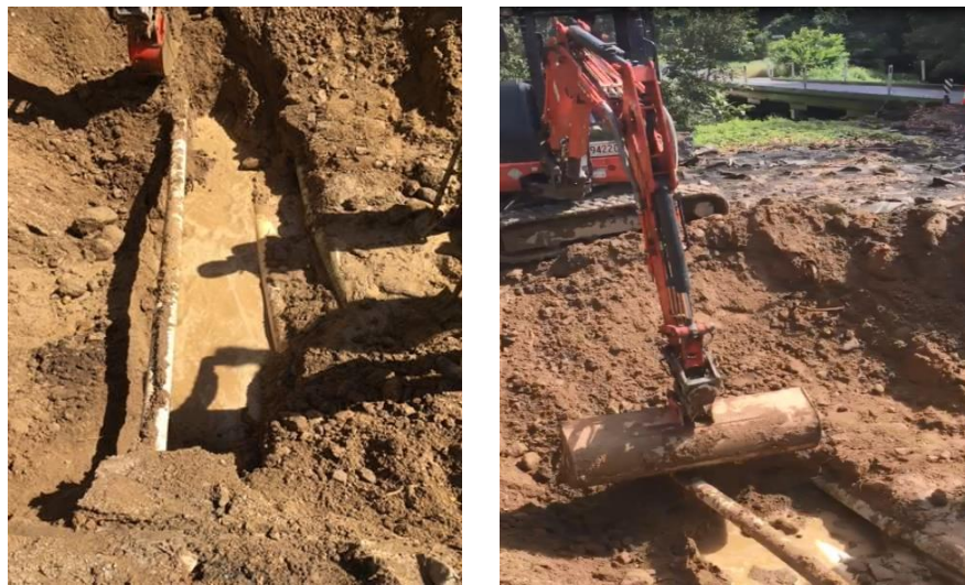
Water main break in Whyanbeel
