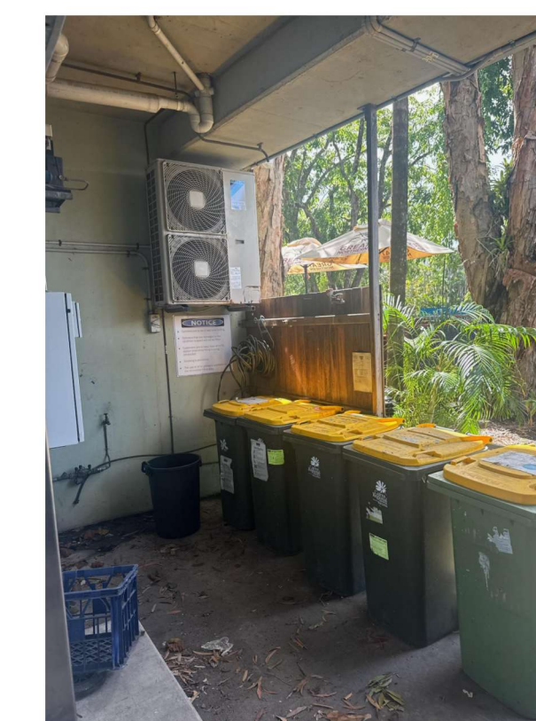
EXISTING WASHDOWN HOSE COCK
