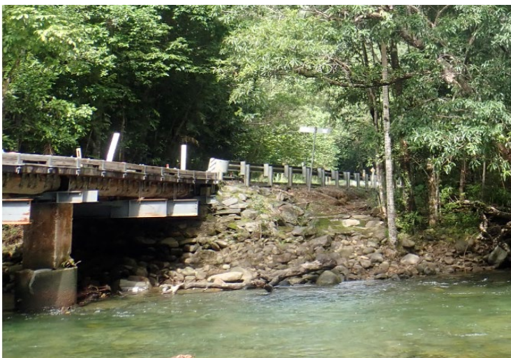
Southern abutments at mid-tide. Bank is almost vertical on both sides of the abutments and drop directly into the low flow channel of Noah Creek. Birds cross the road from orchard to Noah Creek Eco-Stay to the south of the guard rails in picture: literally at the driveway
