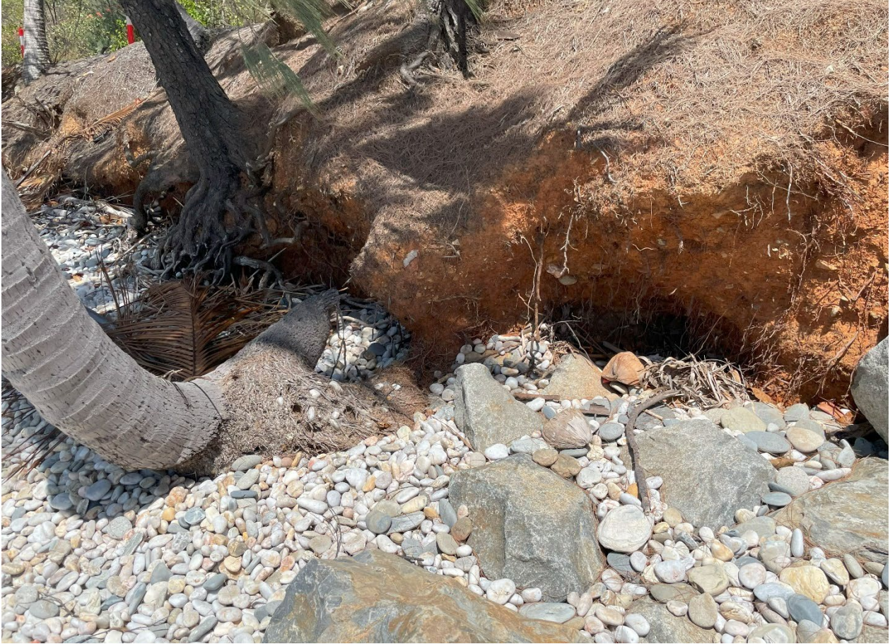
Figure 4-10: Eroding embankment comprises no material consistent with the beach sediments (not the source).
