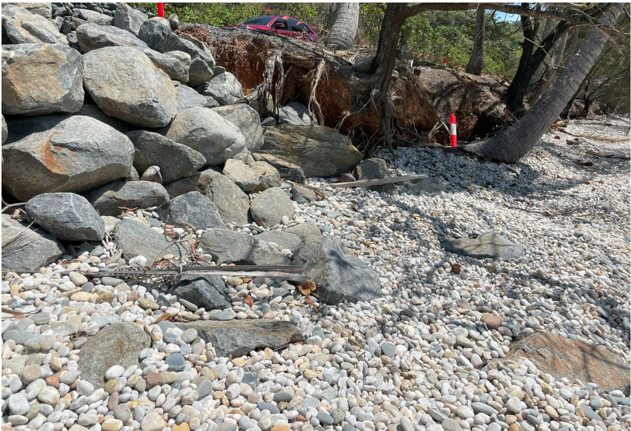
Figure 6-5 Pebble beach berm pushed up similarly in front of eroded embankment and emergency rock wall
