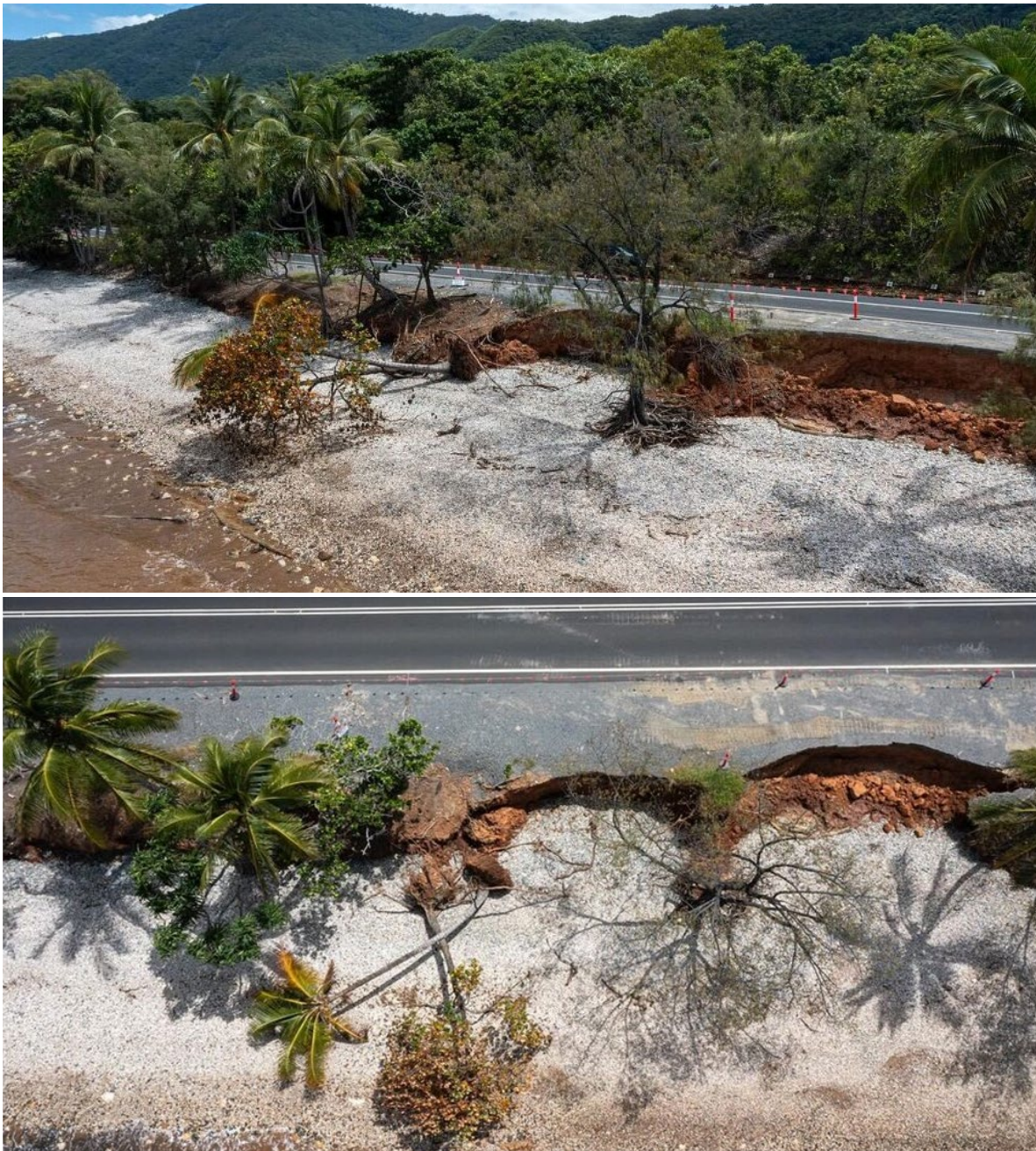
Figure 1-1: Damage to embankment at Pebbly Beach due to Cyclone Jasper
