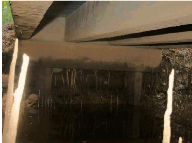
Erosion exposing the abutment under Lutra Bridge
