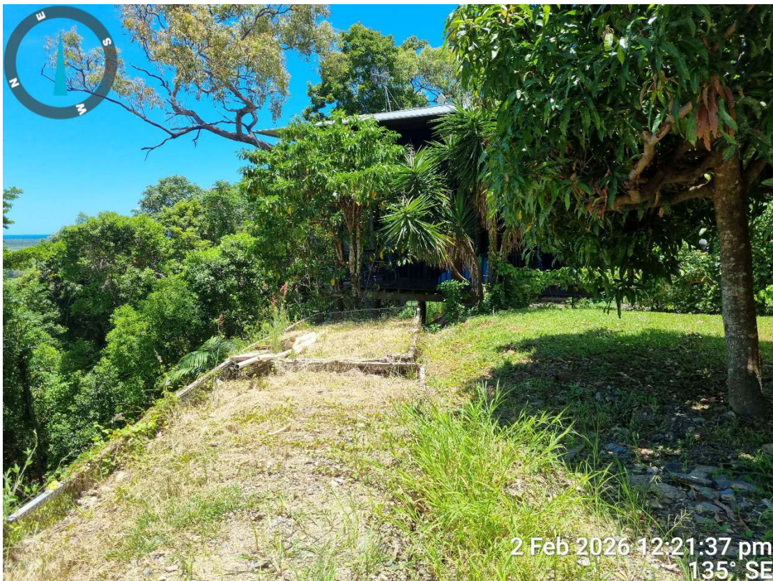
PHOTOGRAPH 3: View of ground slumping behind upper row of cane bins
