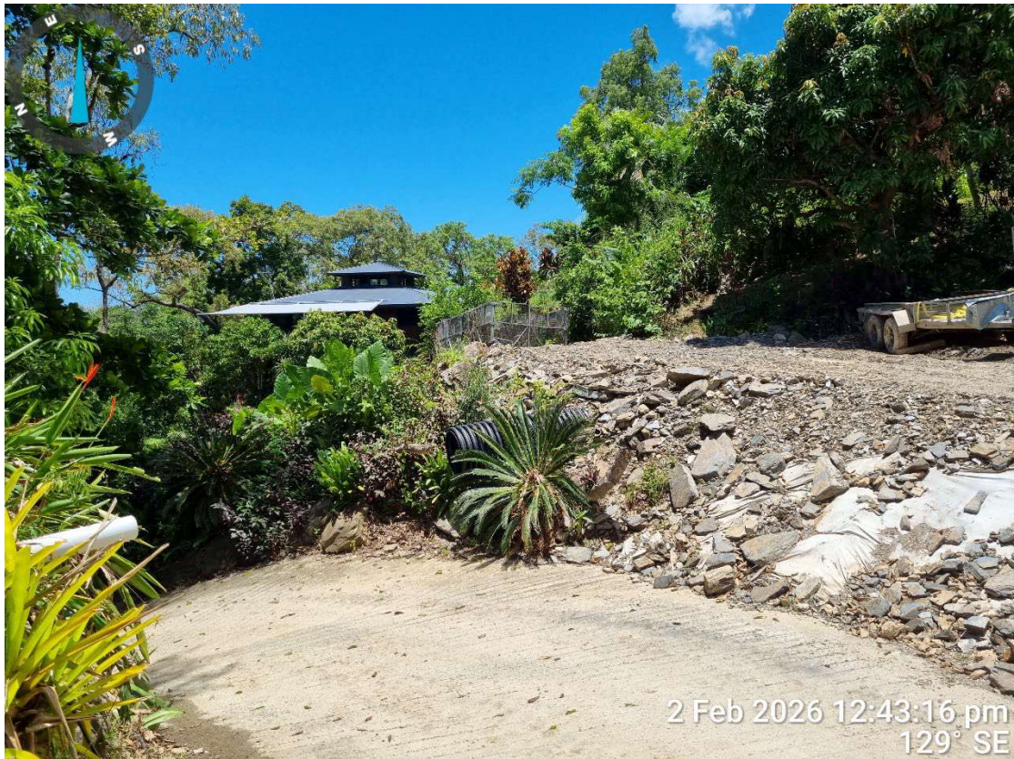
PHOTOGRAPH 6: View of temporary diversion drain and uncontrolled fill
