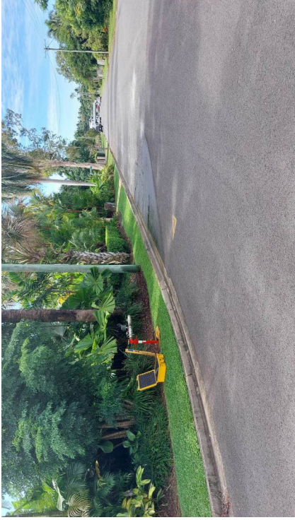
STREET FIRE HYDRANT FH#3
