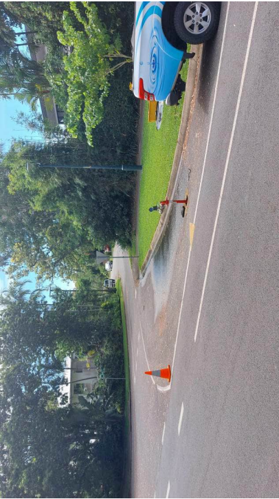
STREET FIRE HYDRANT FH#1
