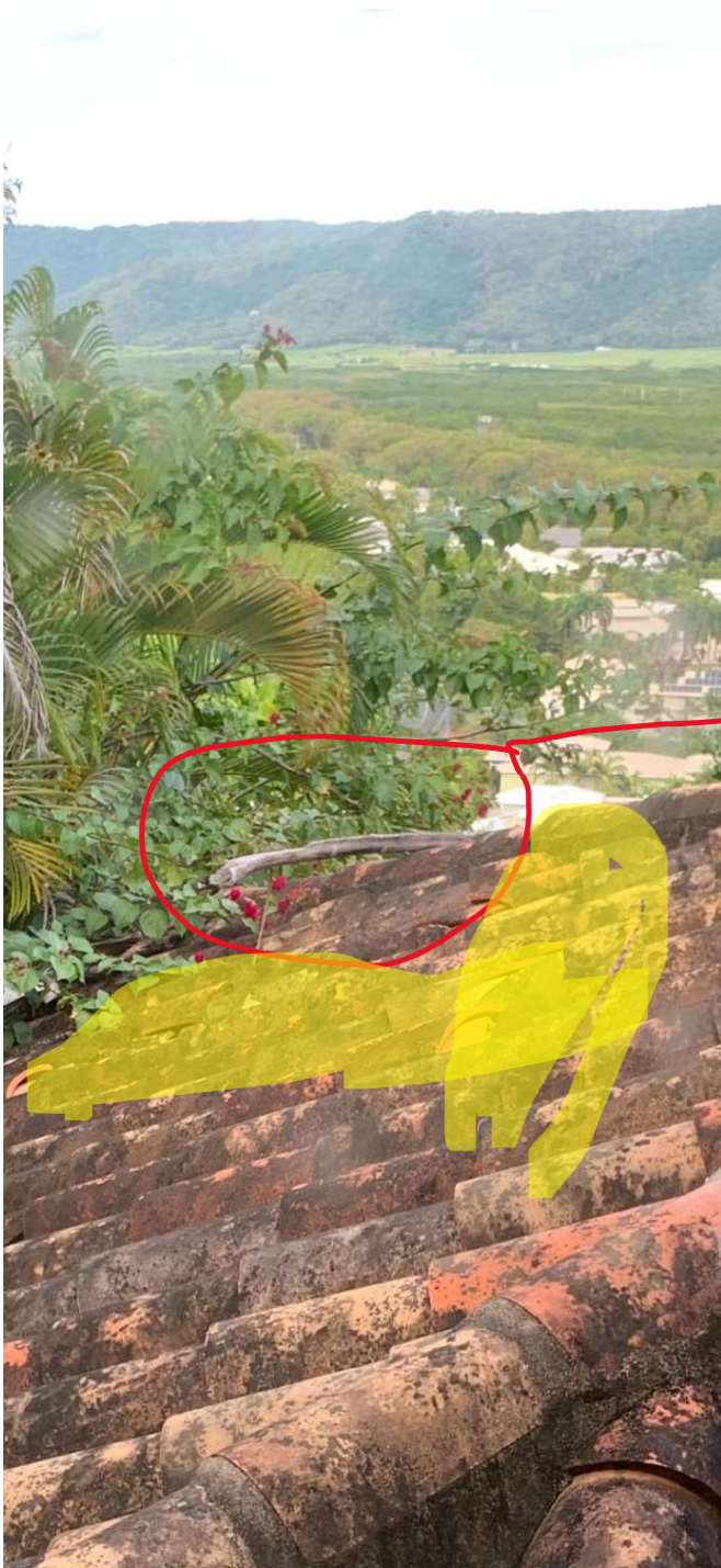
Photo 2 - 44 Island Point Road Roof tiles – Broken and evidence of Palm Frond landed on roof
