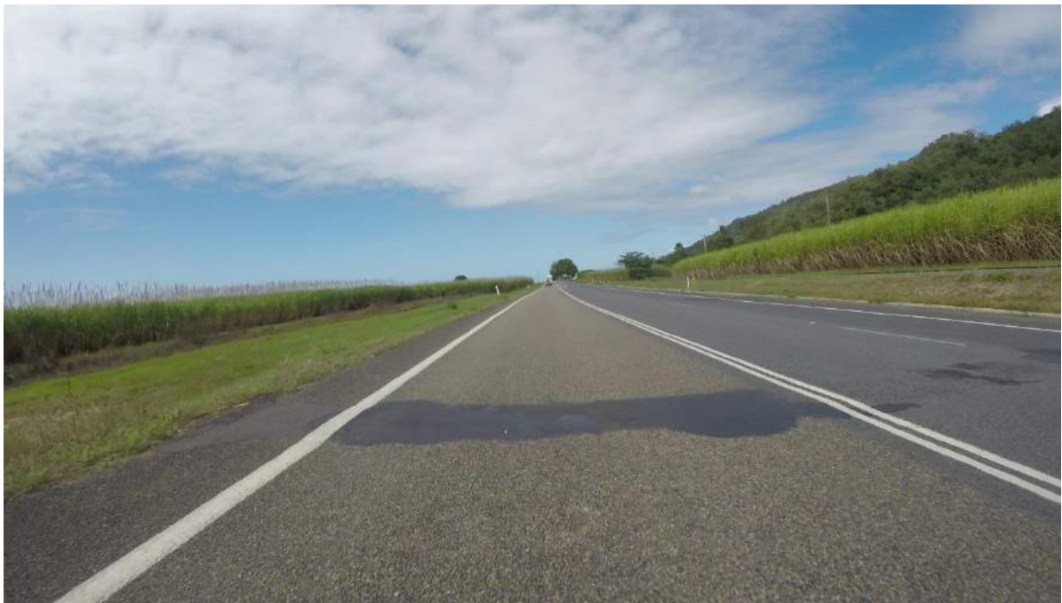
Pavement Deformation at 900m
