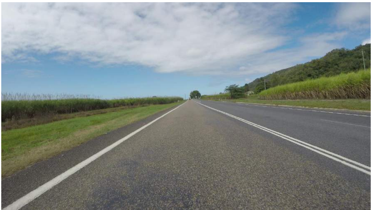
Flushing found at: 900-1000m
