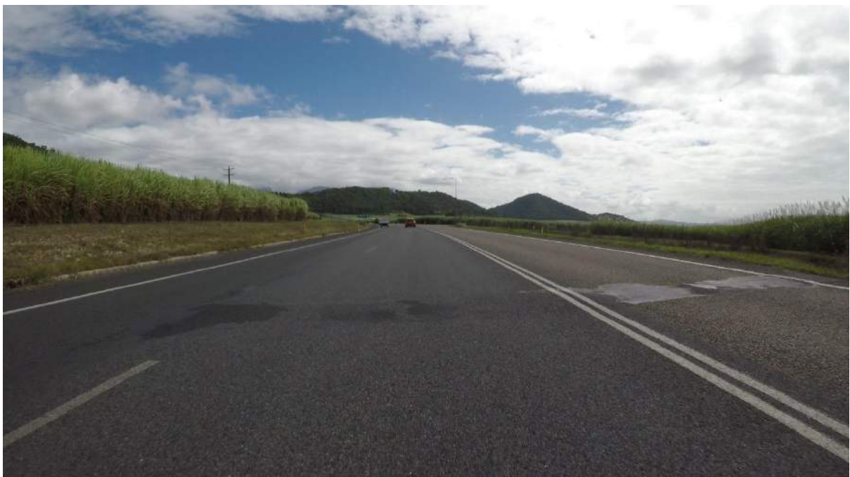
Pavement Deformation (road crossing trench) at 2700m
