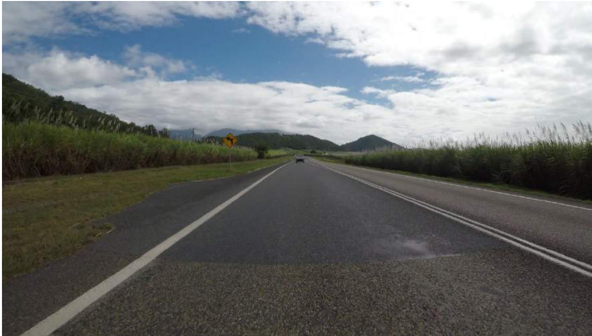
Longitudinal Rutting at 1800m
