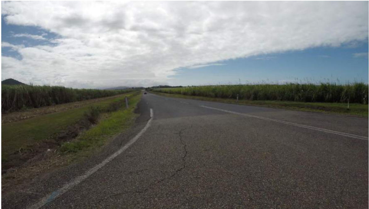
Longitudinal Cracking at 3000m
