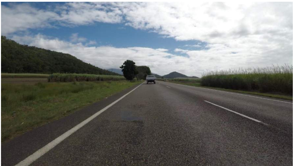
Longitudinal Rutting at 1700m
