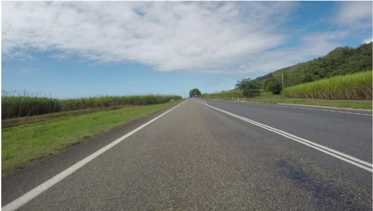
Flushing found at: 900-1000m
