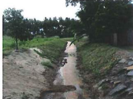
Plate 4. Southern drain looking from culvert at end of Marlin Drive looking east
