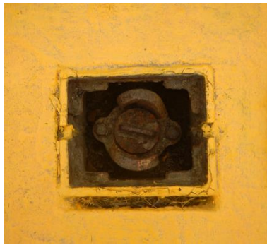
Image of a hydrant plug
