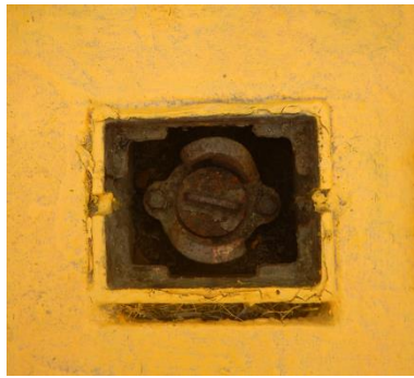
Image of a hydrant plug
